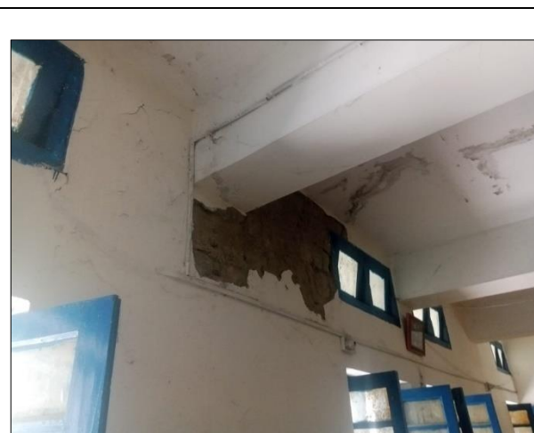
Figure 5 Damage in Lawari House Boys Hostel Dir College
