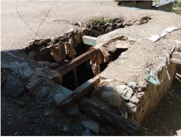
Figure 6 Collapse of a Room in Residential Building at Muhala Kalshow, Dir City
