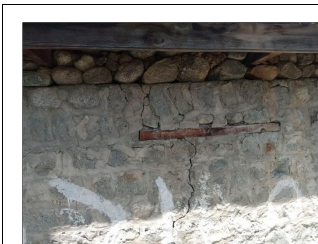
Figure 4 Cracks in Wall of a Residential Building at Muhala Shao, Dir City
