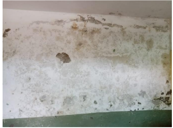
Figure 7 Dampness a Residential Building at Muhala Shao, Dir City
