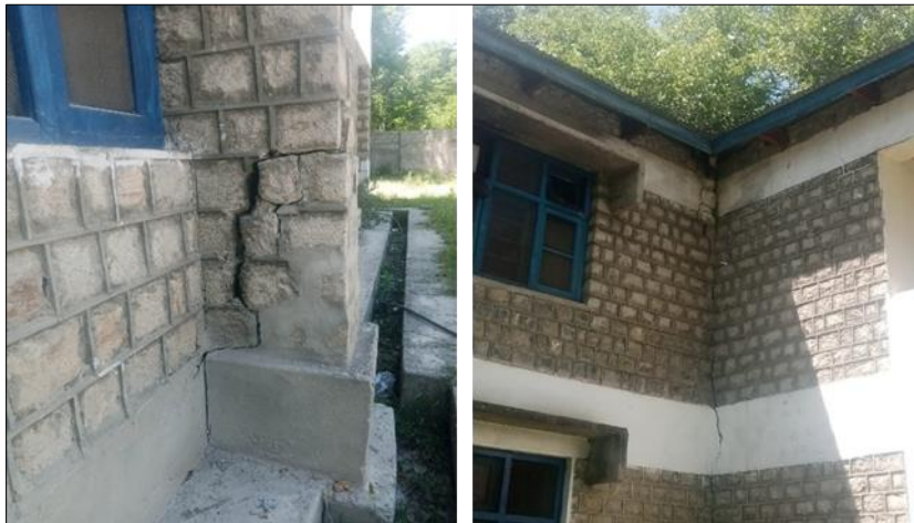
Figure 81 Cracks in Lecturers Hostel Dir College, Dir City
